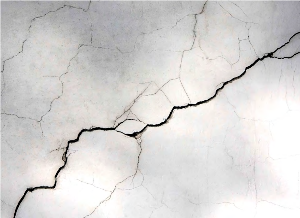
Picture 137 – Wall cracking after exposure to weathering on poor render quality
