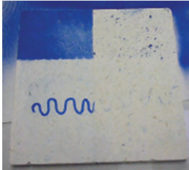
Picture 23 – Anti-graffiti effect on a porous surface. Right half-side is SurfaPore AG and subjected to cleaning under hot-water, without scrubbing.
