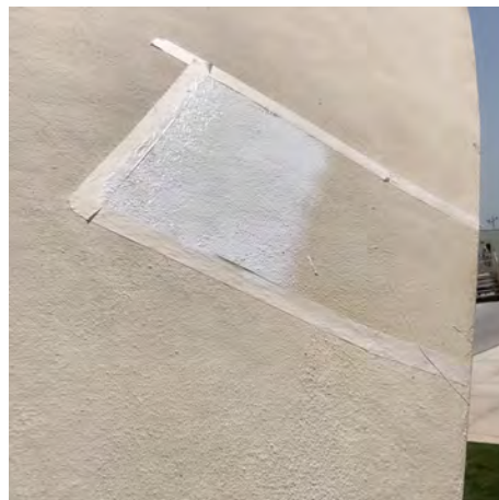
Picture 85 - Application of SurfaPaint SCP Concrete Acrylic Enamel Paint. The sample is exposed for six months on cleaned substrate. Note the difference on whiteness.
