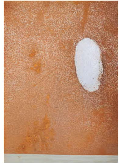
Picture 134 - Final result of rust removal, within 10min of DeSalin Rust Remover application
