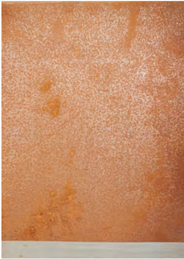
Picture 132 - Rust on a vertical metal surface
