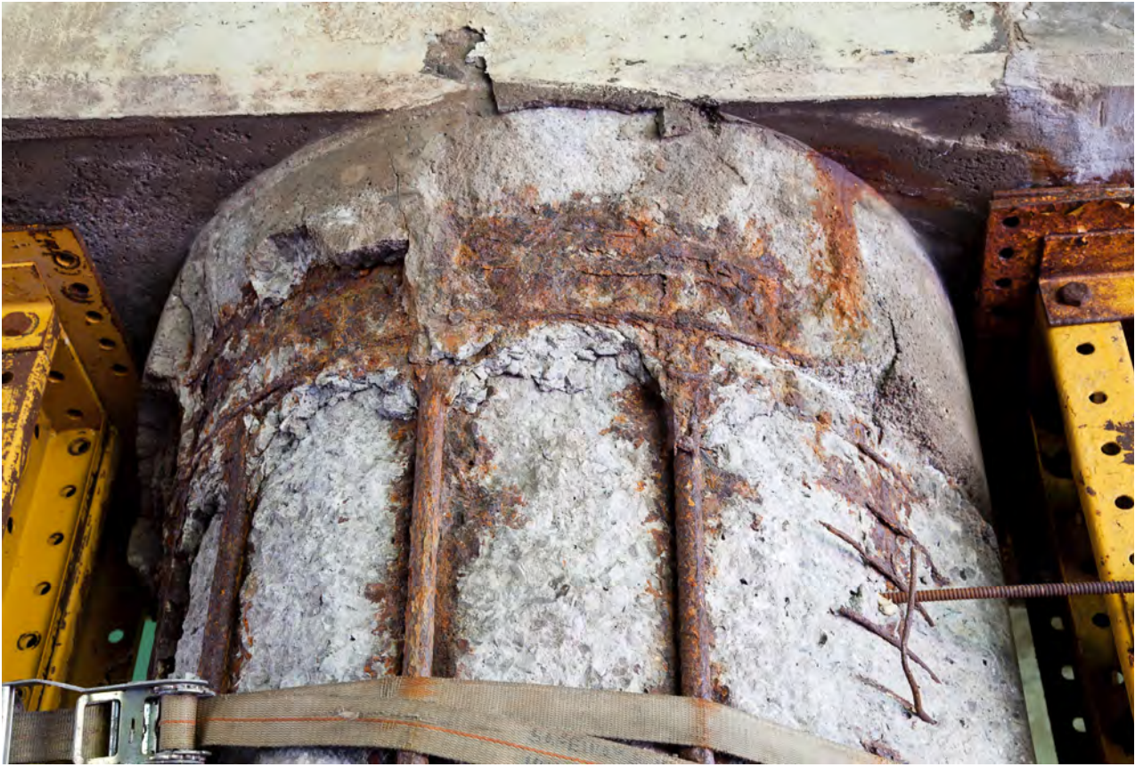
Picture 111 – Carbonation on a bridge cement pillar
