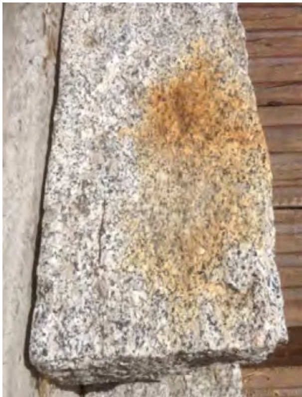
Picture 135 - Rust deposits on a chemicals-resistant granite piece
