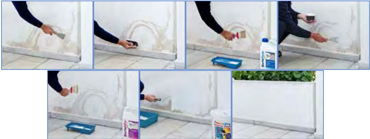
Picture 13 - Reparation sequence for rising damp swelling on walls
