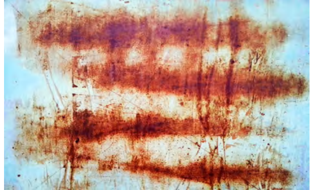
Picture 35 - A typical rusted metal surface requiring restoration and repainting.
