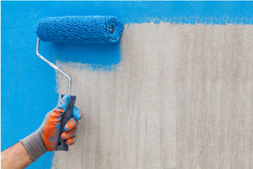
Picture 102 – Application of EPR Epoxy Primer on FeatherPlast AquaX for pool insulation
