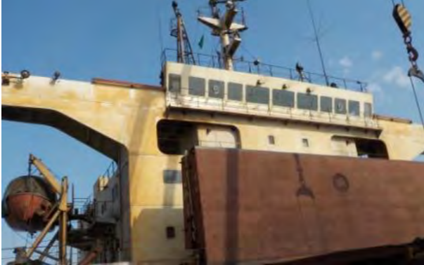
Picture 34 - A typical rusted surface (white superstructure) that blasting and restoration is practically impossible. The application of SurfaGuard RCS can restore and stabilize rust before the application of fresh top coating.
