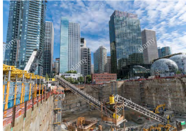
Picture 6 - Foundation preparation works of a skyscraper. On the left side, soil cement base (SCB) has been applied and concrete casting frame has been laid. On the right side the excavated soil base is visible.
