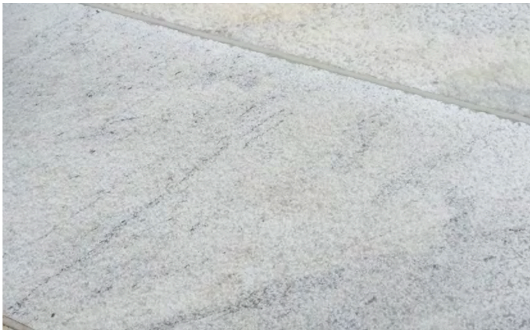
Picture 77 - Application of SurfaPore FX SB on "flamed" floor marbles of Oslo Opera House, Oslo, Norway
