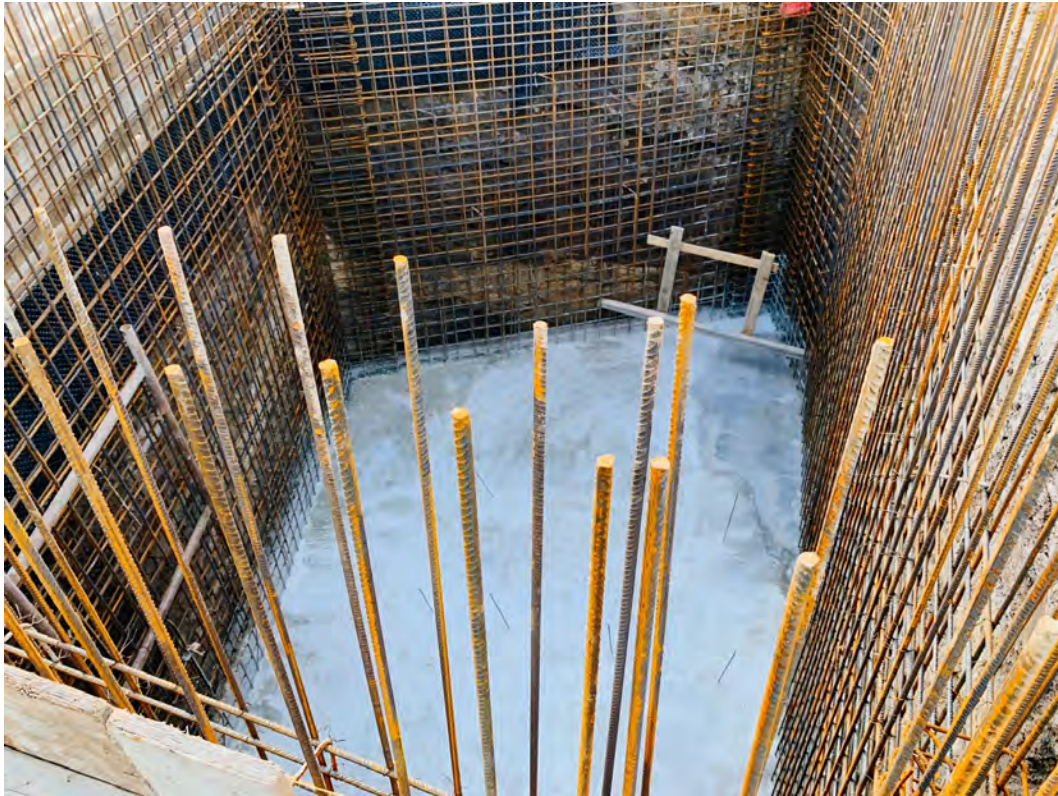
Picture 110 - Septic tank preparation for a residential building in Greece. The reinforced concrete tank has to be perfectly insulated to prevent leakage to the neighbouring buildings.
