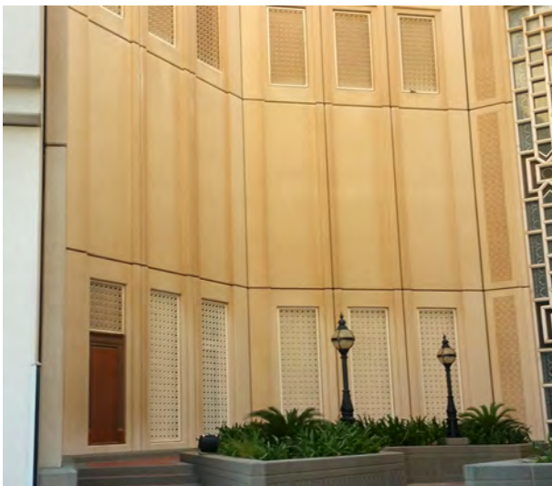
Picture 143 - A palace made of cementitious rendering. Note the dirt accumulation.
