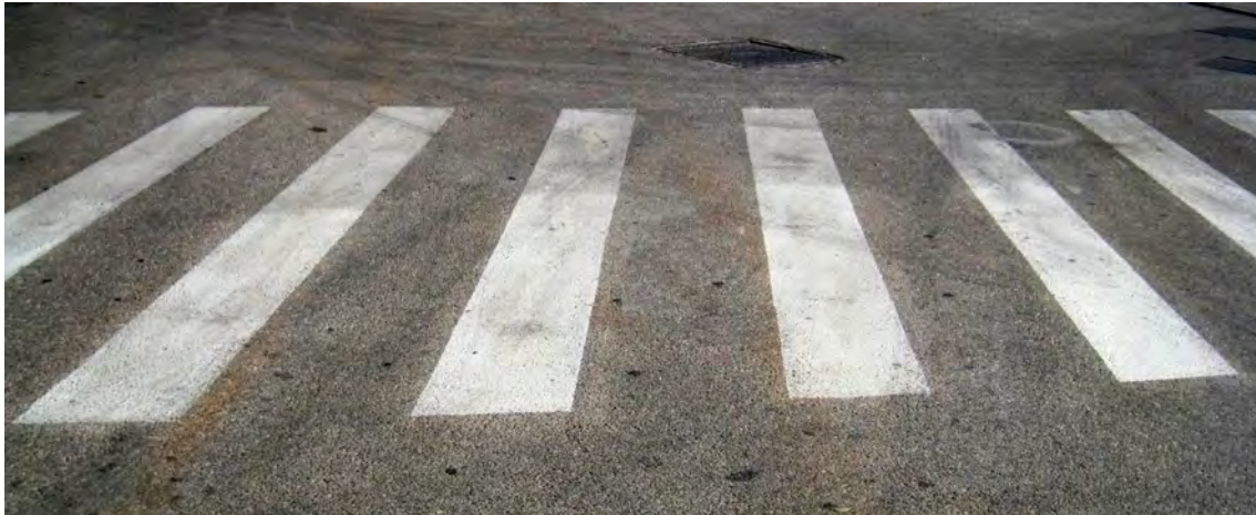
Picture 138 - The effect of SurfaShield C on a heavy-traffic pedestrian zebra crossing, three months after treatment. Upper side is the original road traffic paint, while the lower part has been treated with SurfaShield C.
