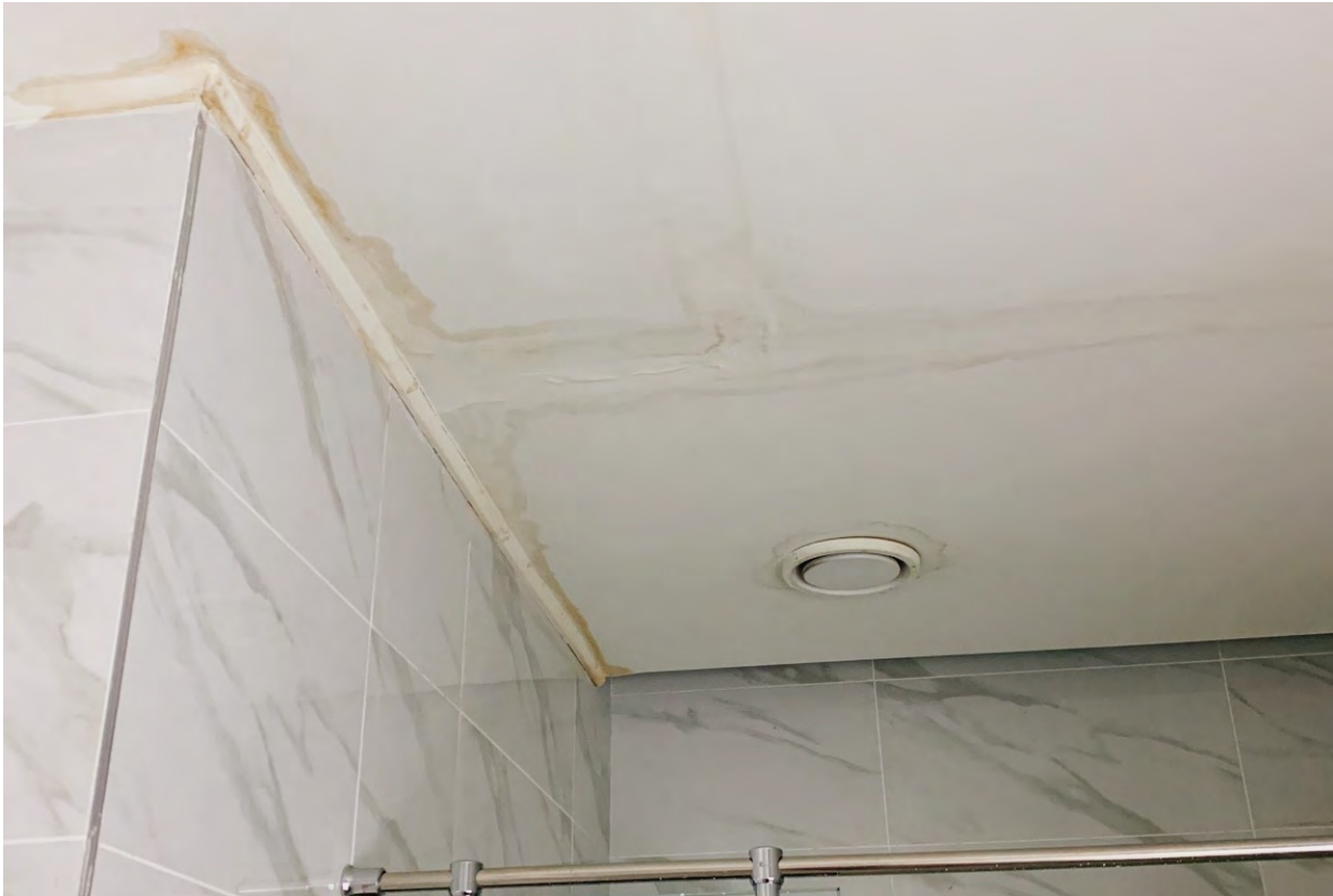
Picture 71 – Non-waterproof drywalls installed on the rooftop of a shower room. Heavy damage would have been avoided by the use of SurfaPore F
