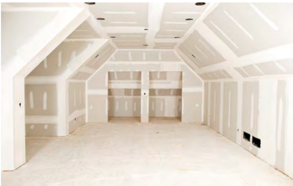
Picture 72 - Application of SurfaPore F as a primer on drywall, before the application of paint
