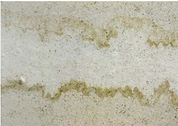
Picture 43 – Old cementitious plaster stabilization (middle bright section). Salt decay and humidity attacks have been eliminated.
